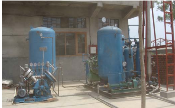
Biogas scrubbing unit and Compression unit at 200 bar
