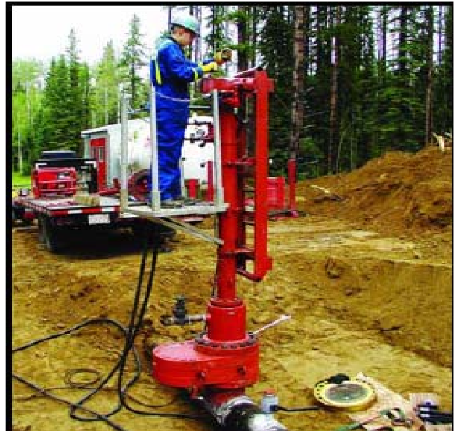
Certified Williamson Industries Technician performing a hot tap with a 760 Tapping Machine as part of a 12-inches Stopple application.
