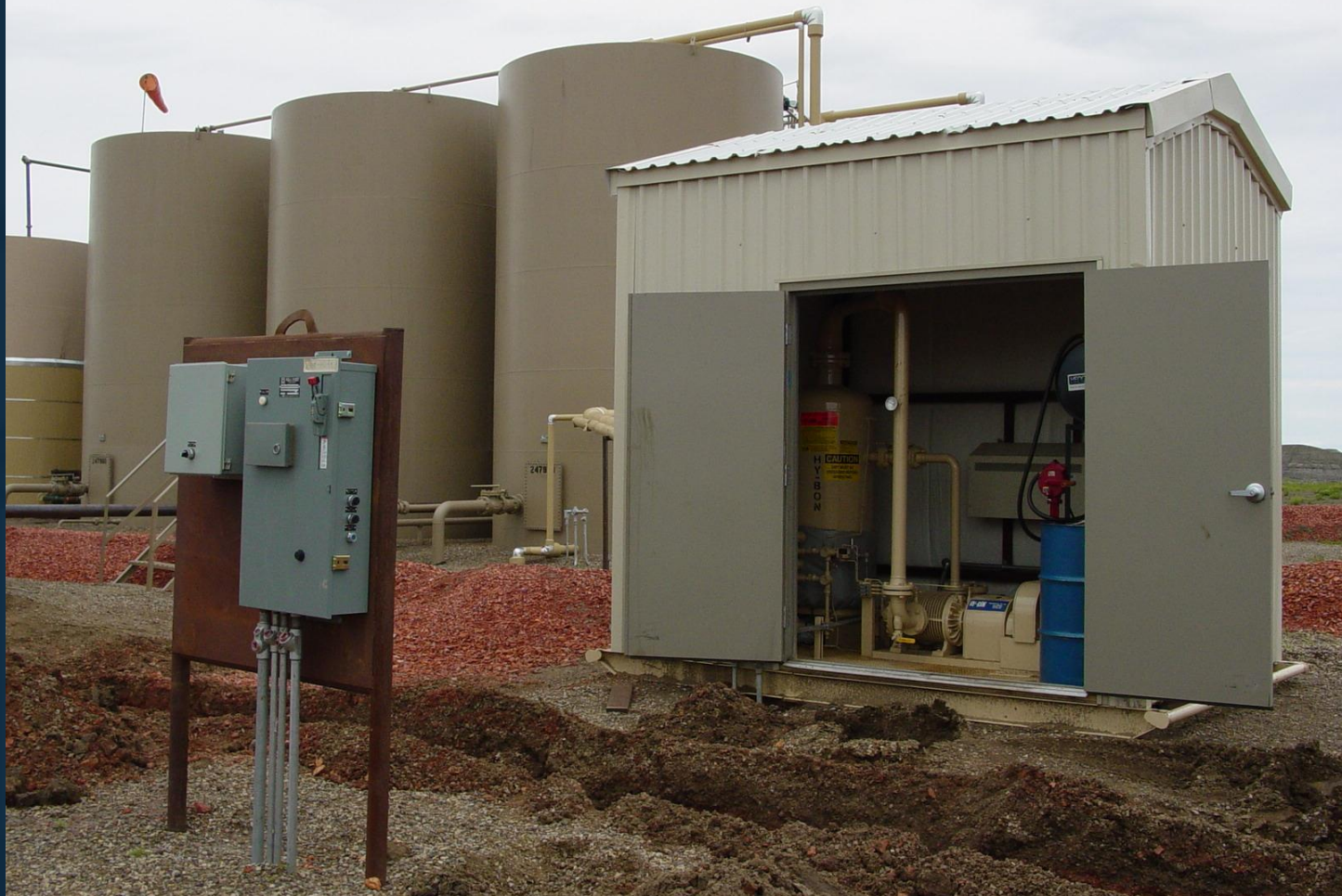
Baker, MT ConocoPhillips VRU installation; Picture Courtesy of Hy-bon Engineering
