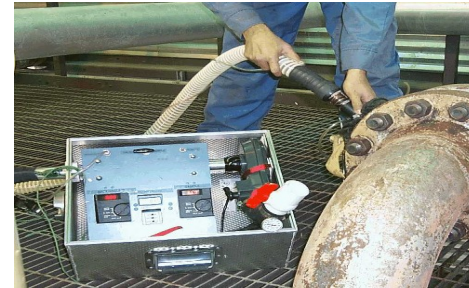
Oil and Gas Systems
