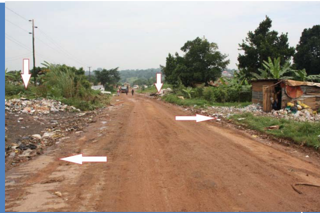
Garbage long Road Before
