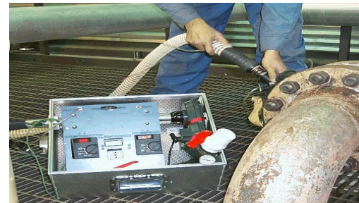
Oil & Gas Systems
