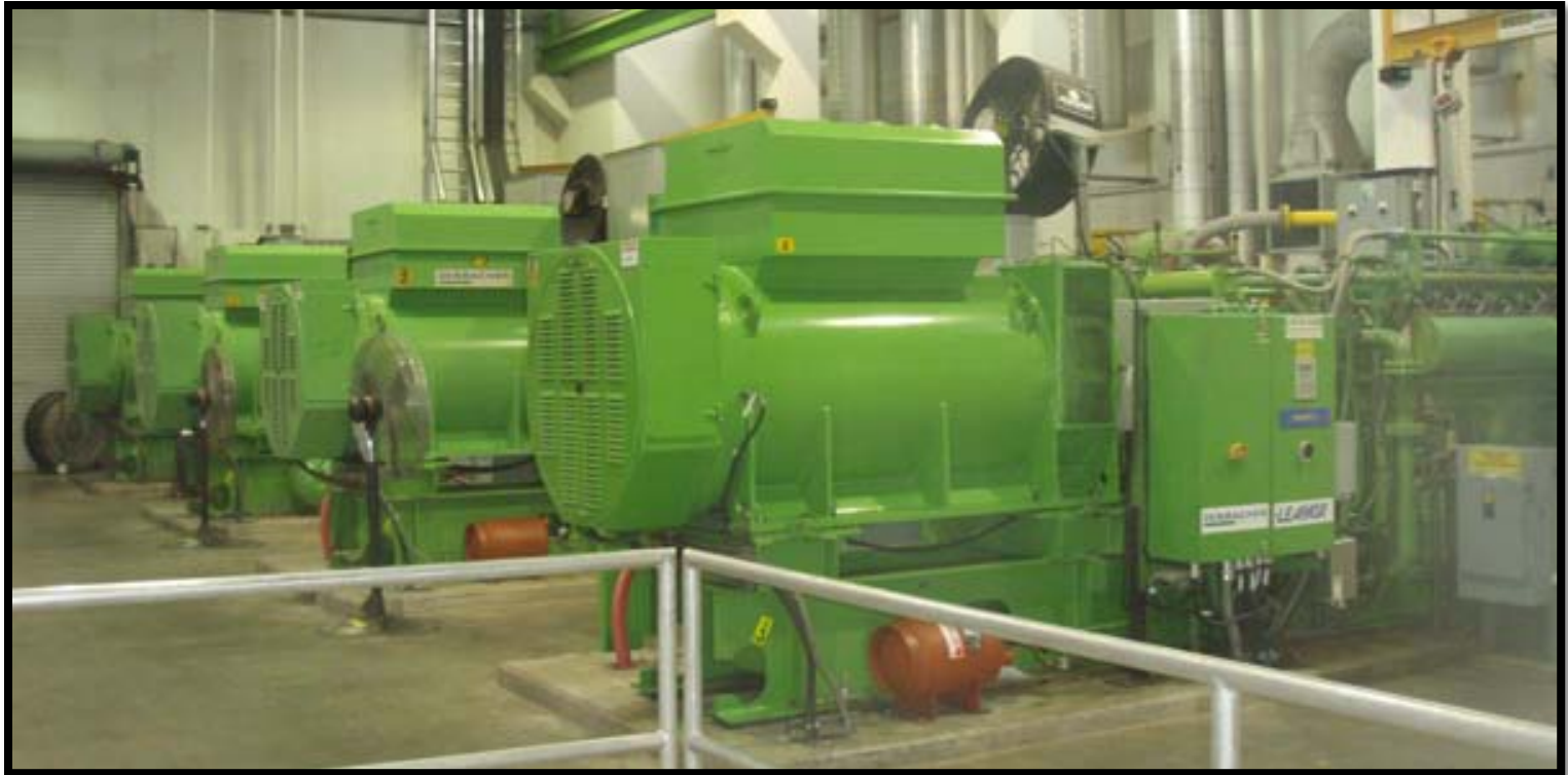
Cogeneration at Annacis Island WWTP
