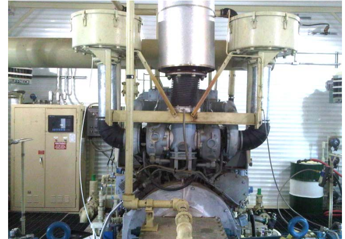
Caterpillar 3512LE - air intake and turbo chargers (rear view)
