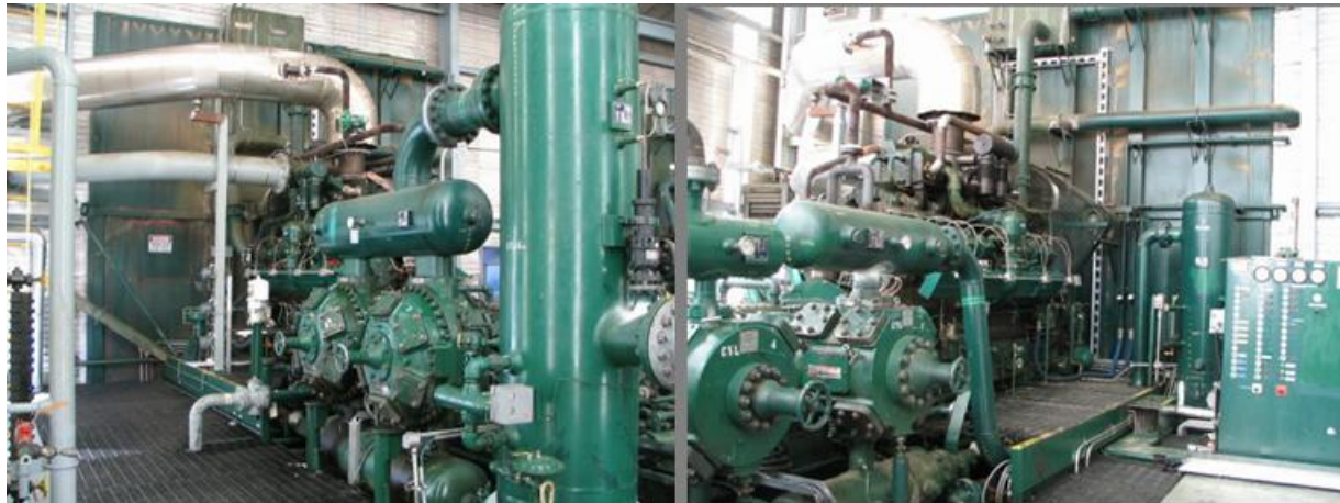
Unit 2 – Waukesha 9390 GSI with REMVue ® Rich-to-Lean AFR
