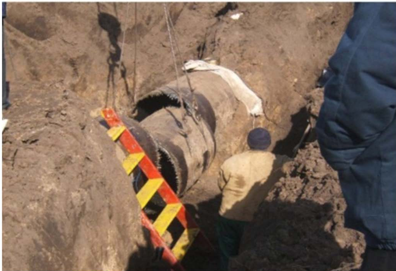
Figure 1: Cutting off the damaged pipeline section – still the predominant repair method in the beginning of 2000 th
