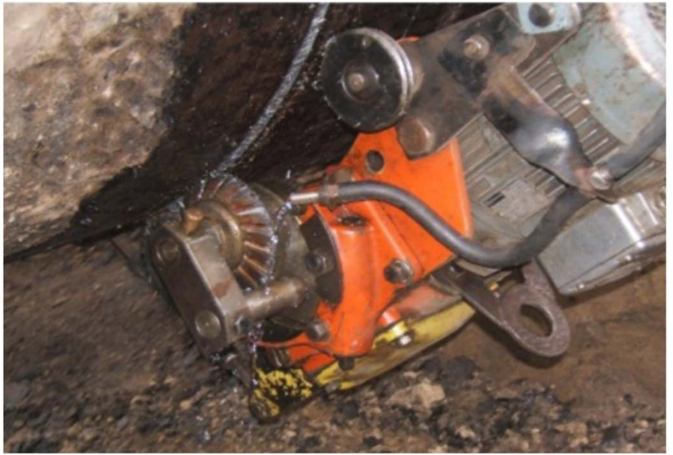
Figure 1: Cutting off the damaged pipeline section – still the predominant repair method in the beginning of 2000 th
