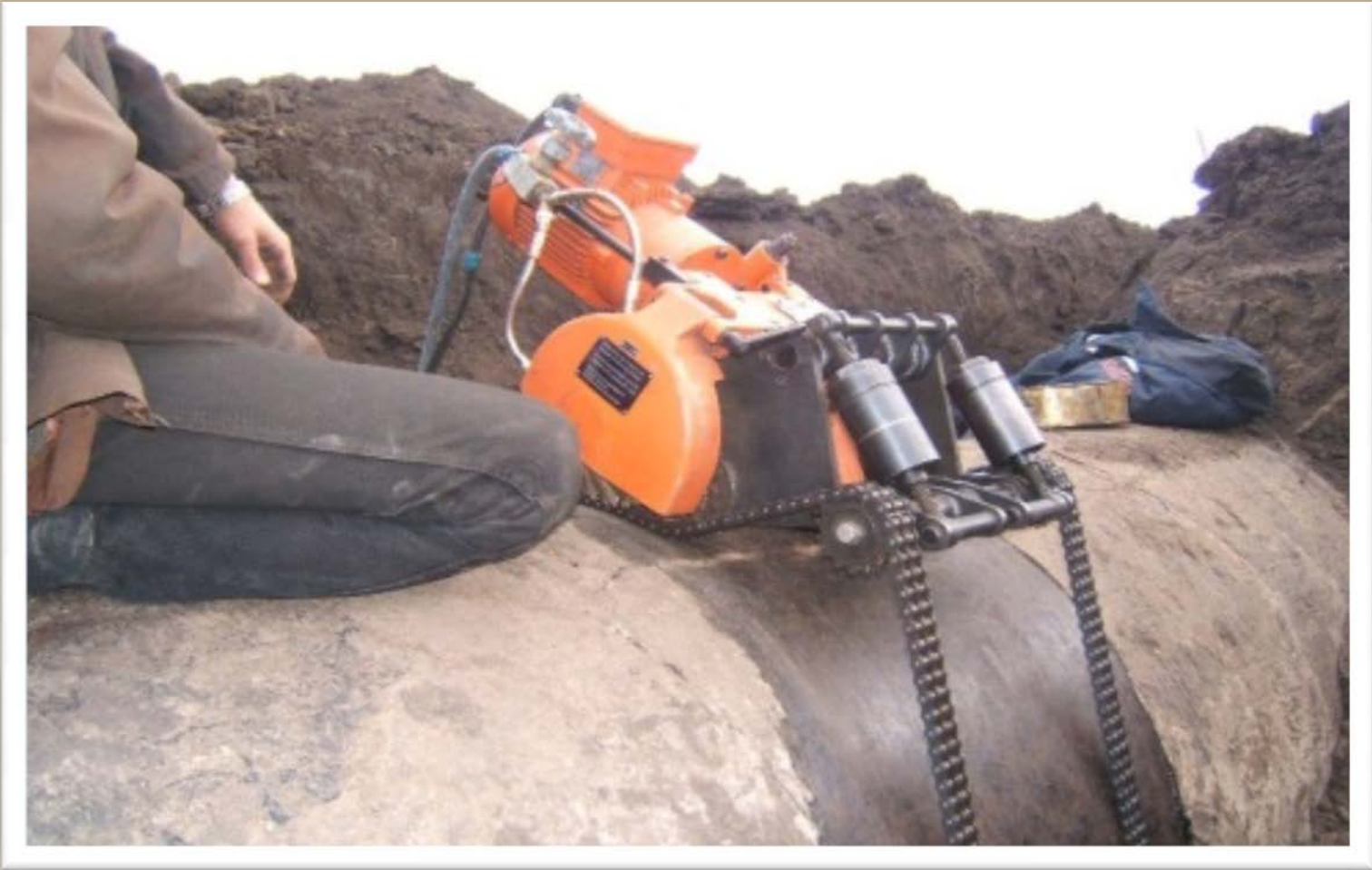
Figure 1: Cutting off the damaged pipeline section – still the predominant repair method in the beginning of 2000 th
