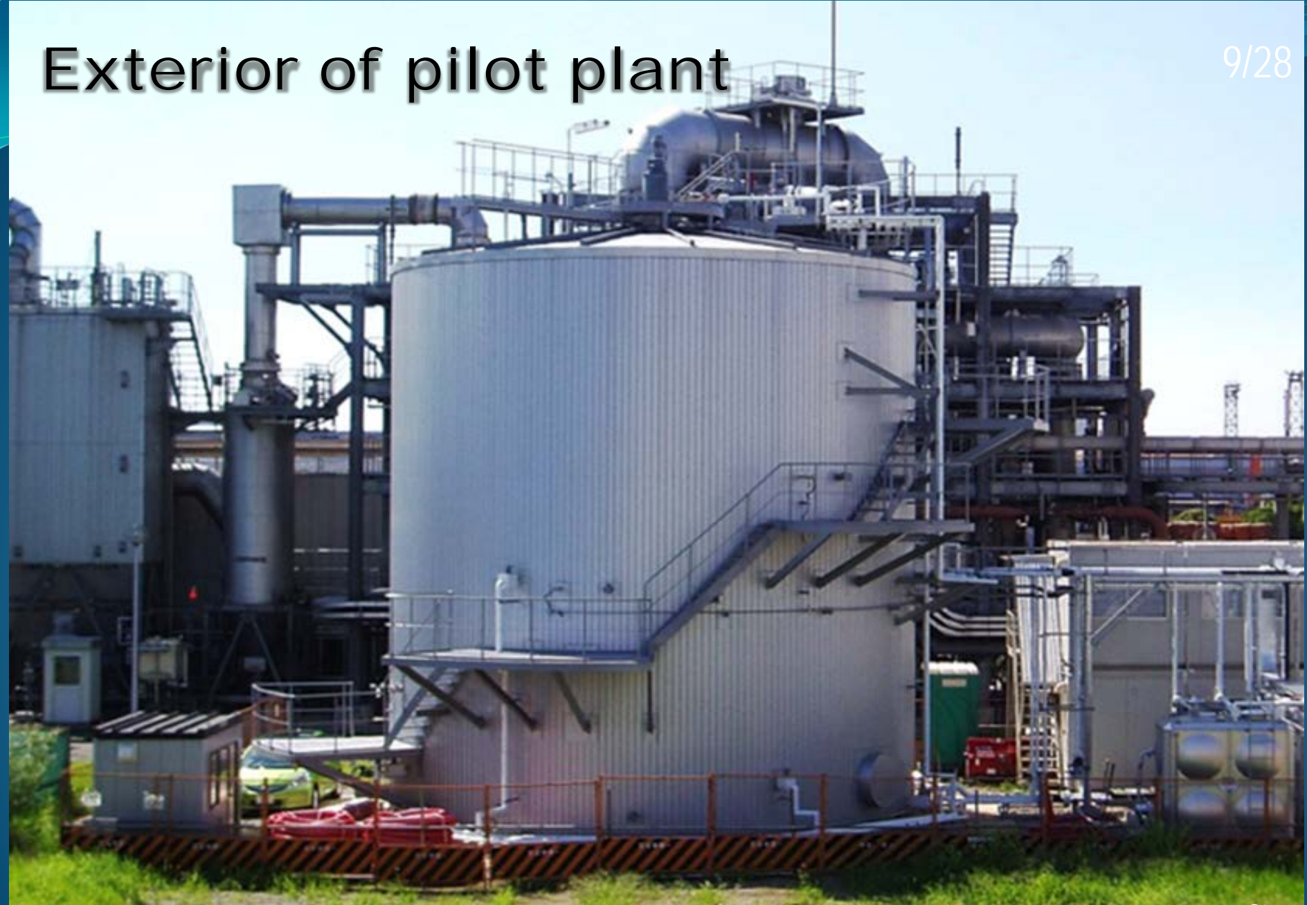
Photograph: Exterior of steel plate digestion tank (capacity: 750 m 3 )
