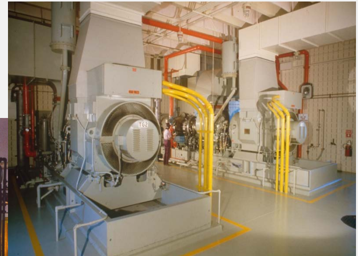
Solar 3 MW Gas Turbine Milwaukee, WI
