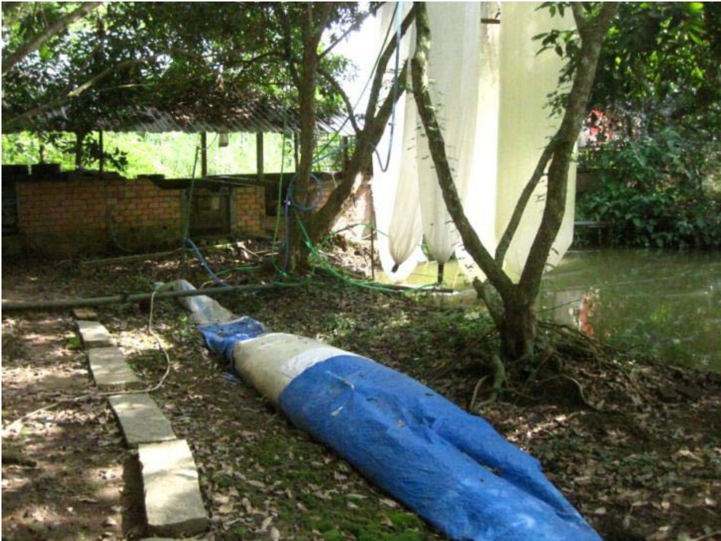
Bag digester (blue) and gas storage bags (white). Polyethylene is low cost construction material.
