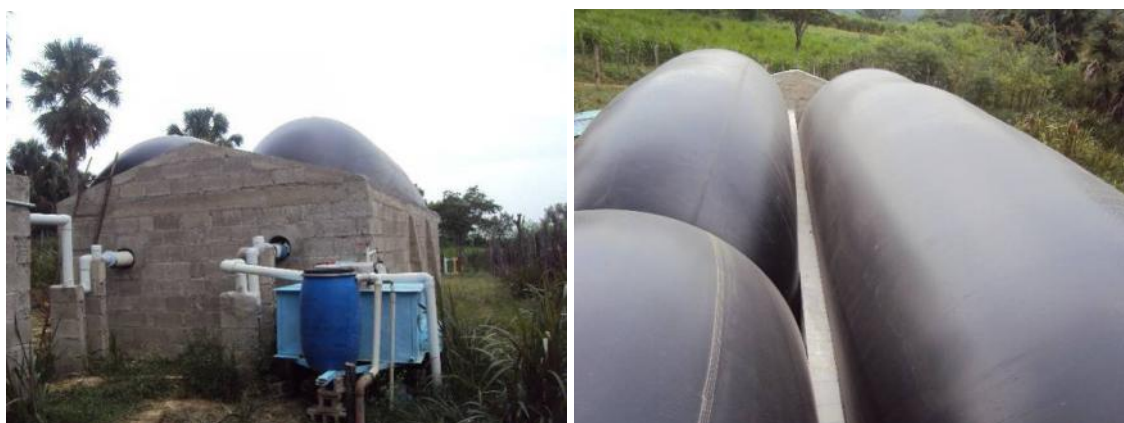
Figure C.1 – Bag Digesters installed by Bioenergym in a Cassava Processing Plant
