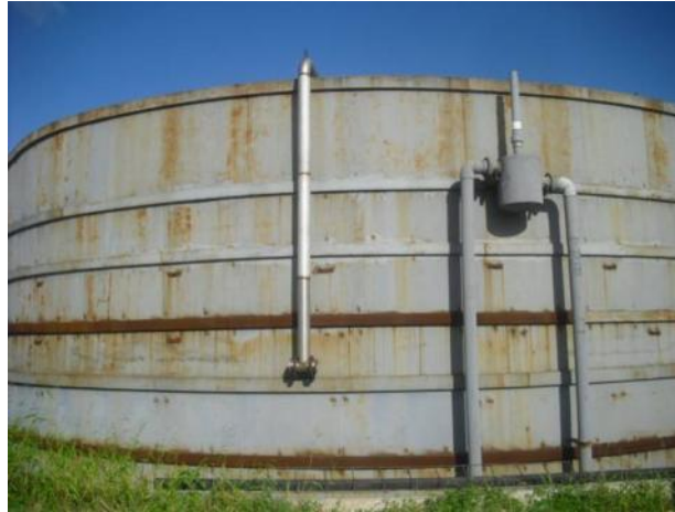
Figure 2.1 – One of the Three UASB Digesters at La Isabela
