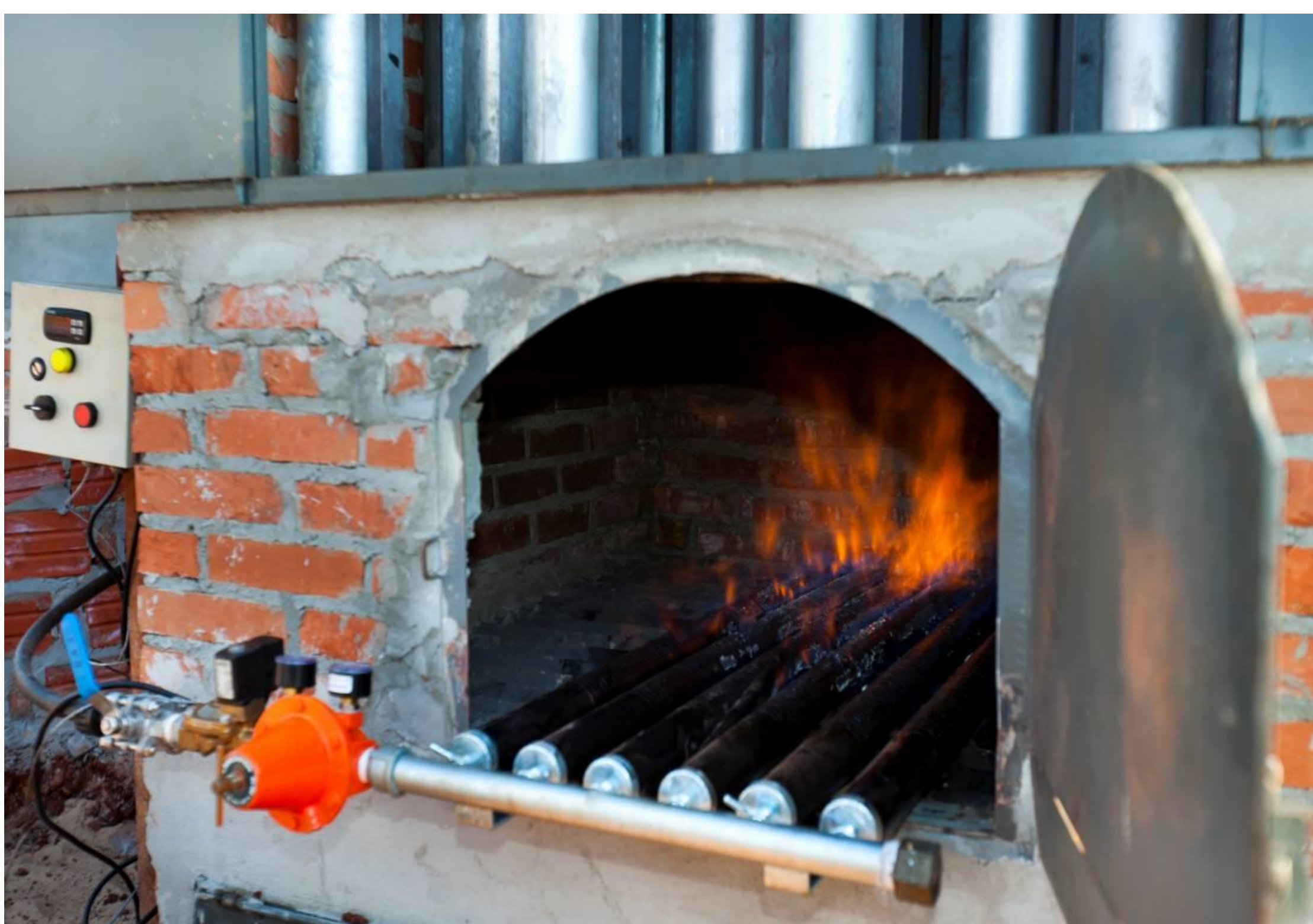
Biogas Furnace to Dry Grains
