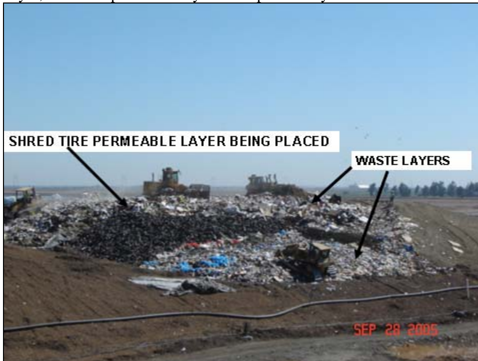
Figure 8. Construction of permeable layers at the Yolo County Central Landfill, California, USA. Photo shows placement of lower waste layer, shred tire permeable layer and top waste layer
