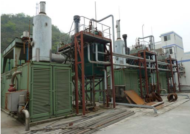
Jenbacher Gensets, Yanjing Mine, China
