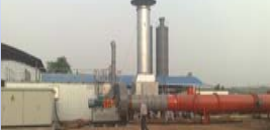
Abatement/hot water ZhengZhou, China
