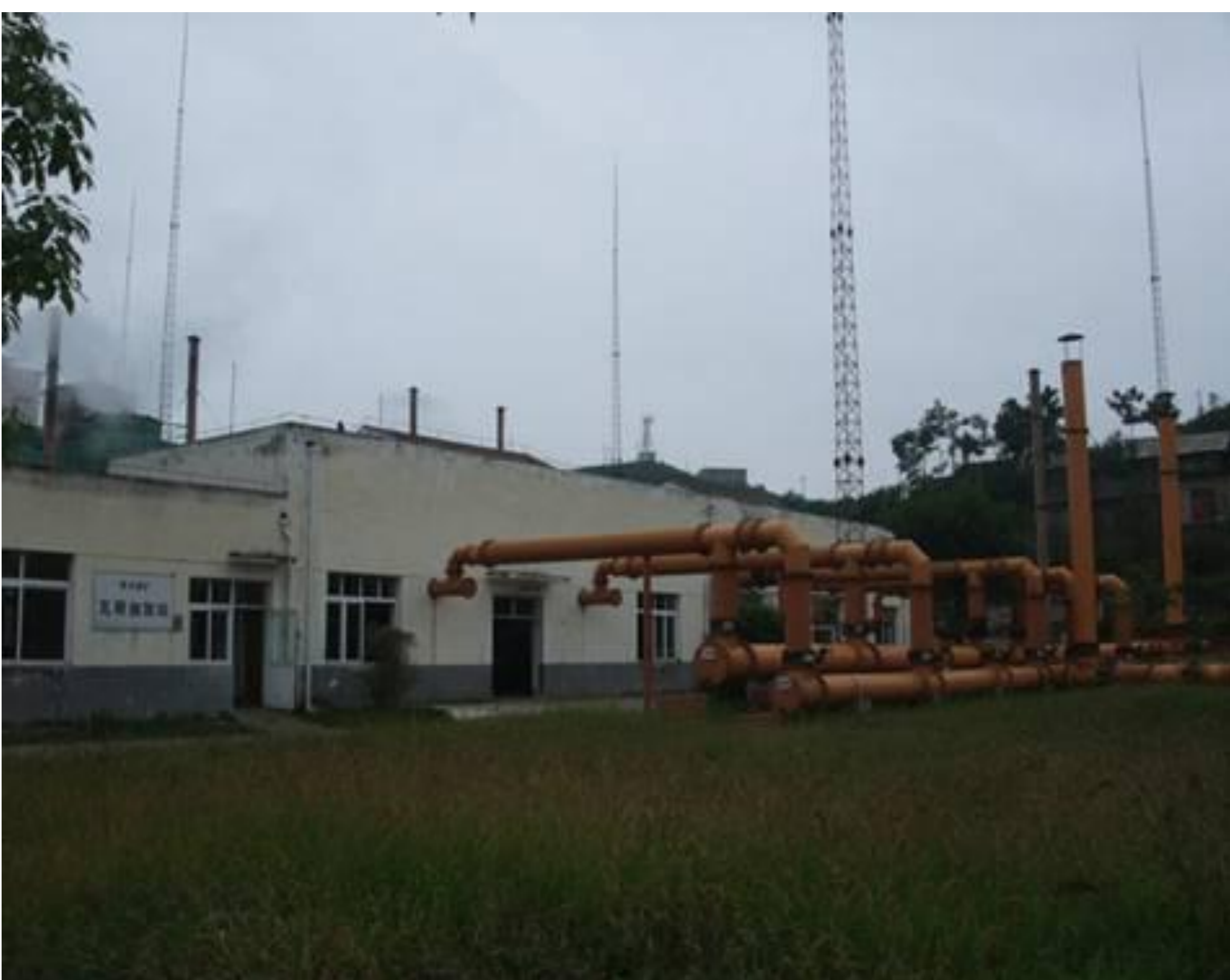
Pump station in Qinglong Coal Mine
