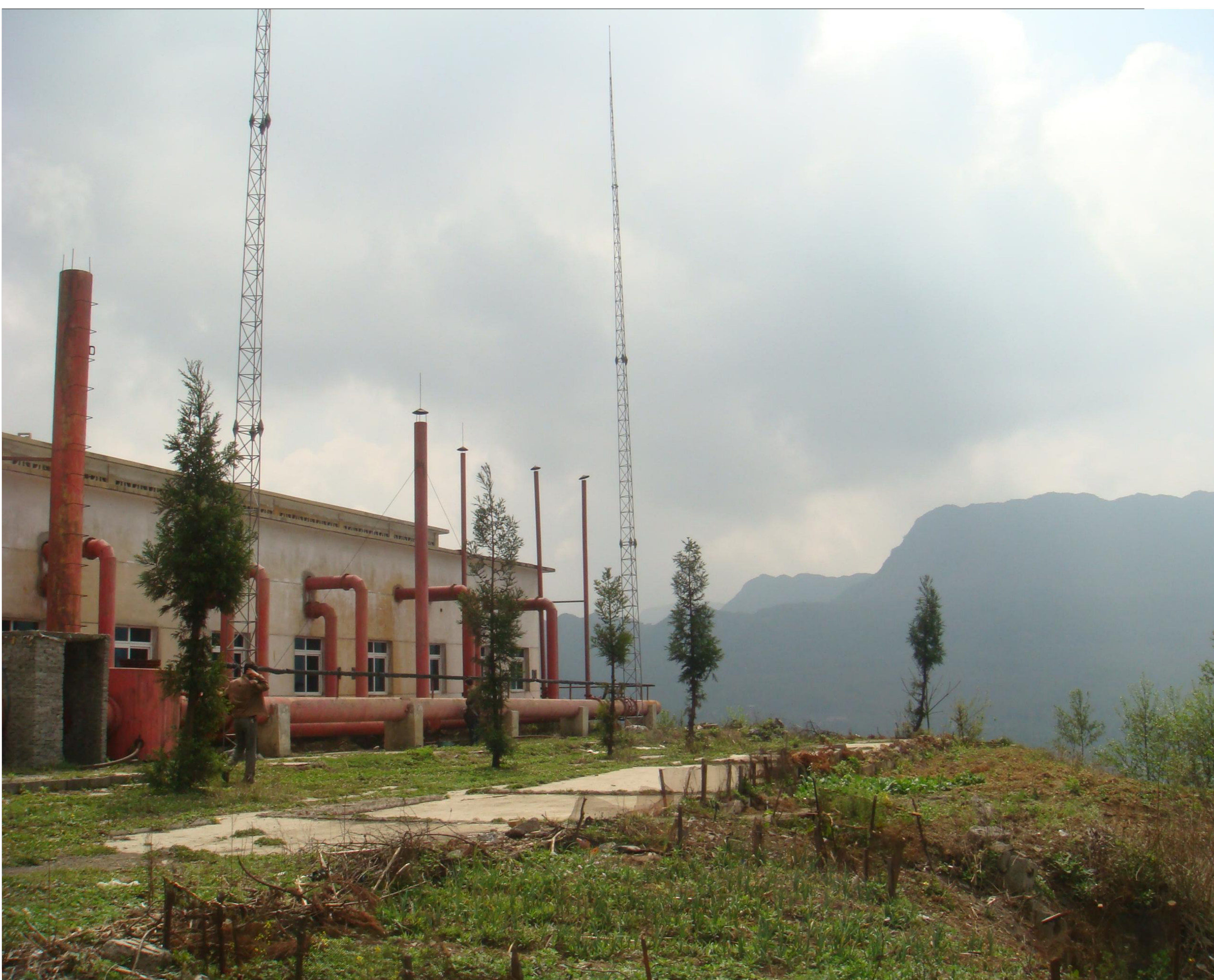
Pump station at mining area 12, Zhongling Coal Mine
