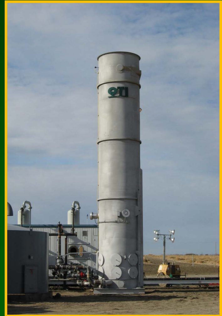
Kerrobert, Saskatchewan Q3000 Incinerator Unit
