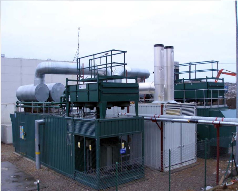
LFG & CHP Plant - Mława
