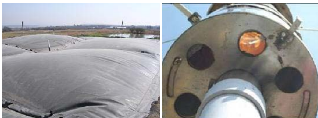
Figure 2.3 – Panoramic View of Santa Mónica Digester (left), Flame in the Chimney (right)
