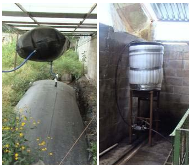
Figure 2.2 – La Joya Digester (left) and Heating System (right)
