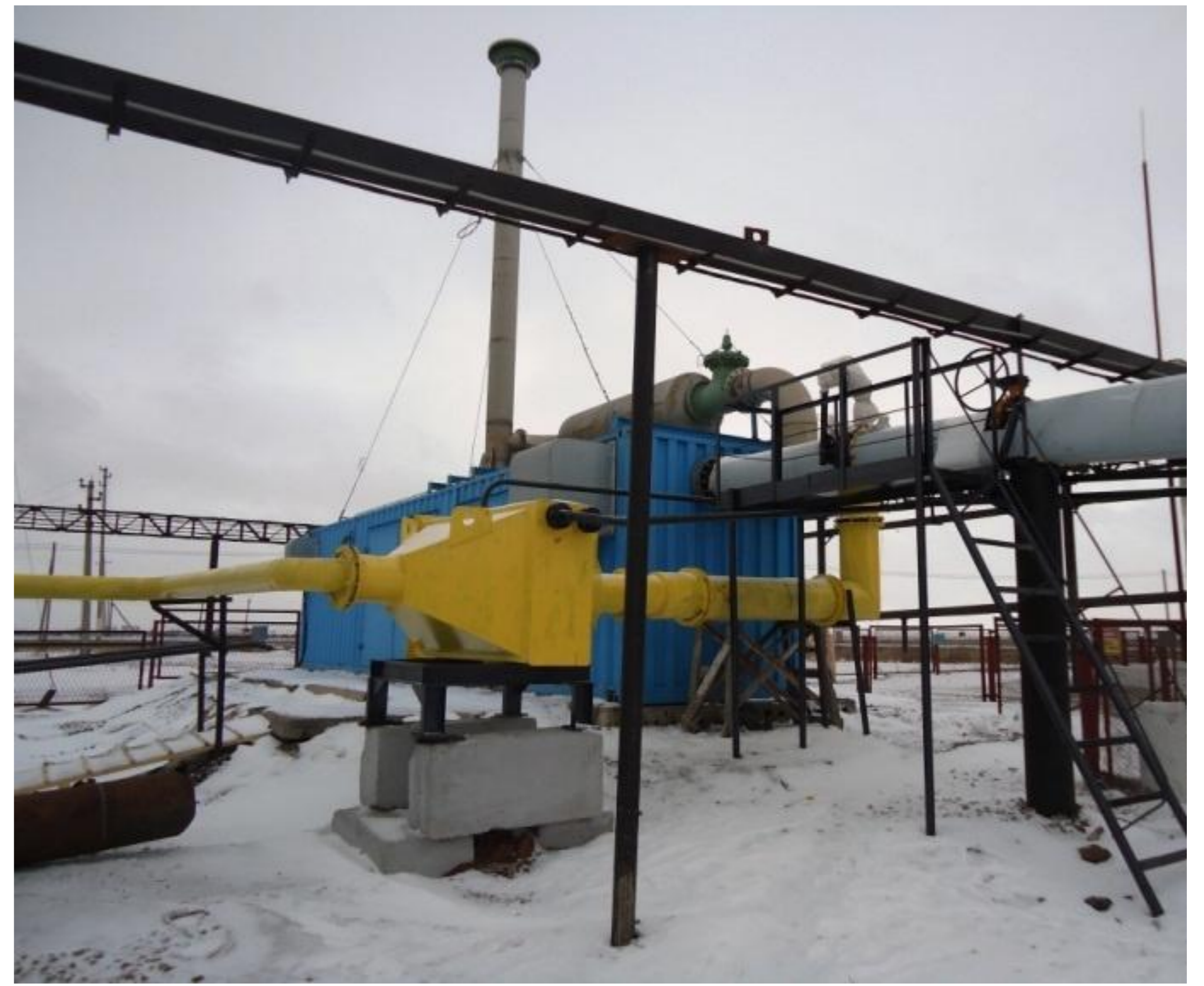
Methane Extraction Plant and Gas Cooler
