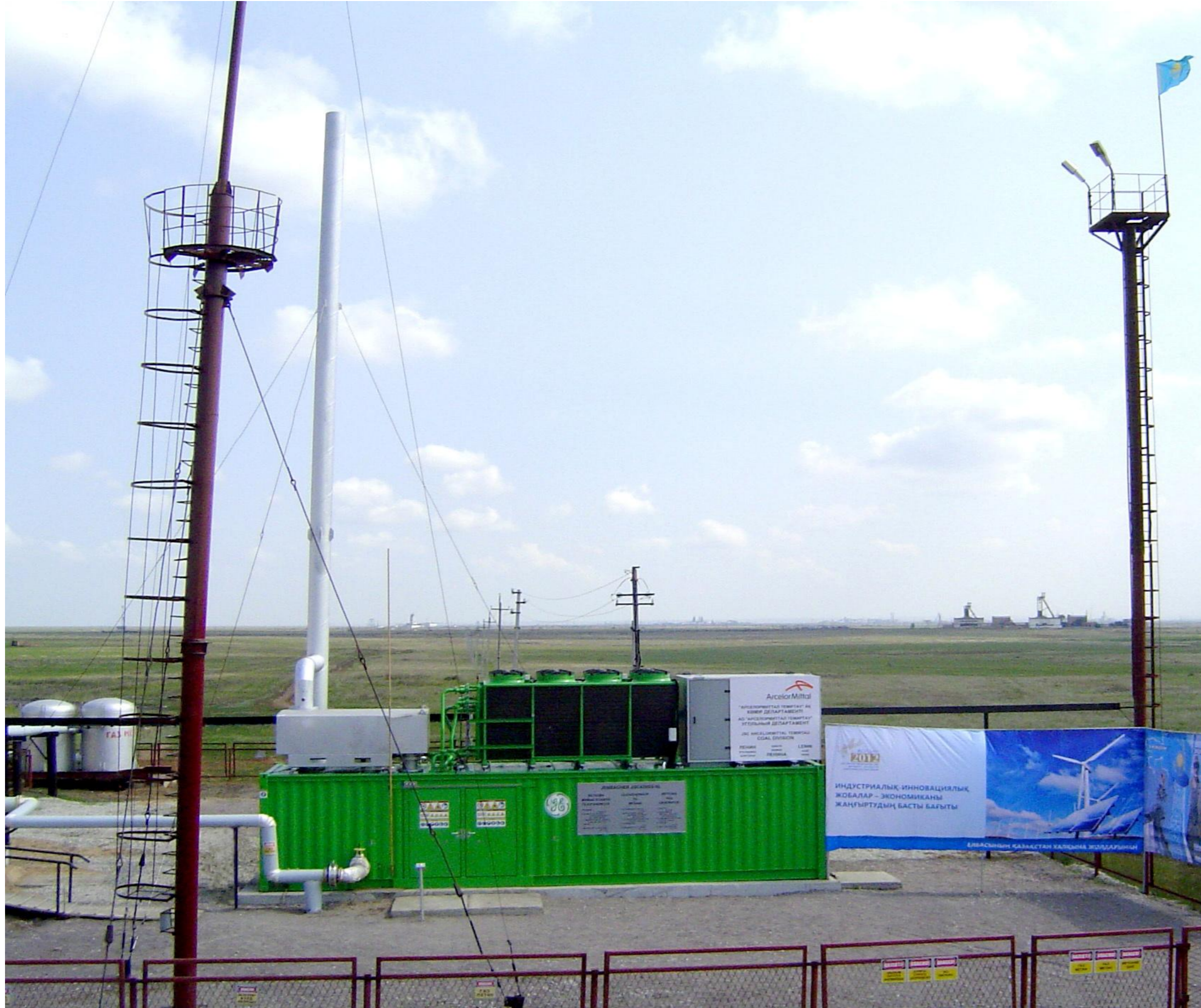
Containerized Gas Generator Set at Lenina Mine
