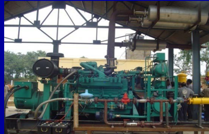
CMM Based Generator
