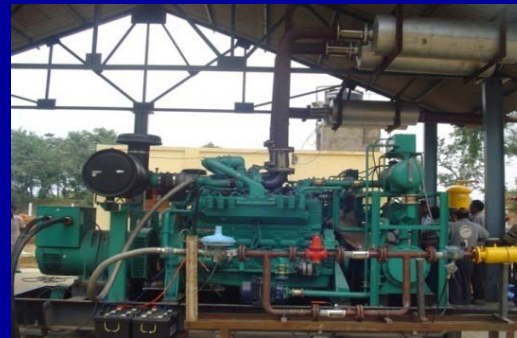
CMM Based generator
